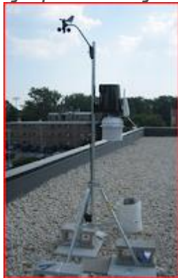
Σταθμός VP2 24hrs fan aspirated radiation shield.
